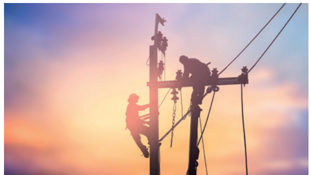
Gridworks, backed by CDC Group, develops and invests in critical on and off-grid power infrastructure in Africa.
